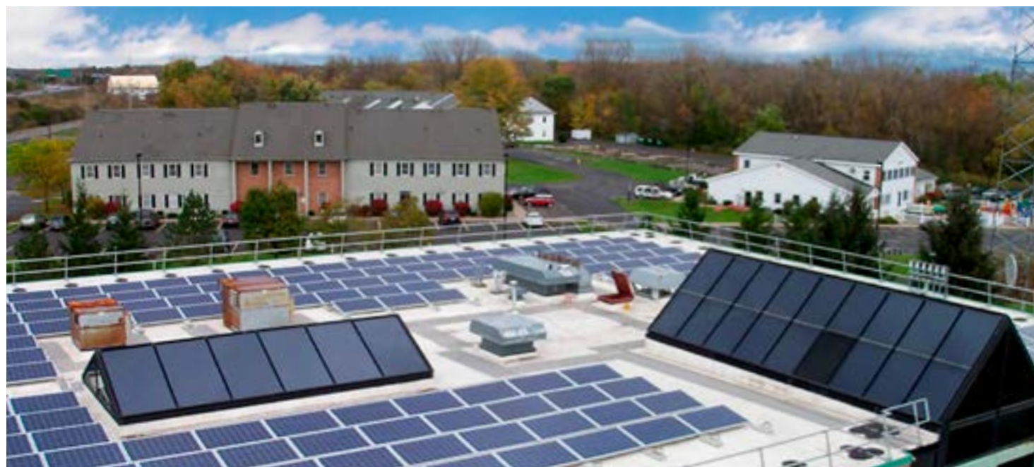
51 KILOWATT SOLAR ARRAY INSTALLED ON THE DEWITT TOWN HALL ROOF (TOWN OF DEWITT)
