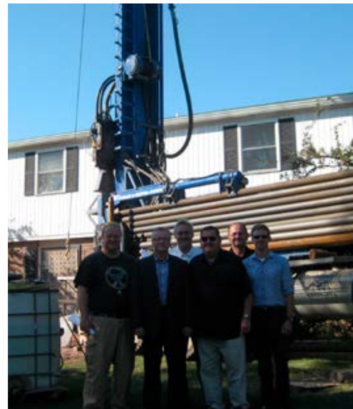
DRILL RIG FOR GEOTHERMAL INSTALLATION AT THE AUTUMN GARDENS SITE (LOCKPORT HOUSING AUTHORITY)
