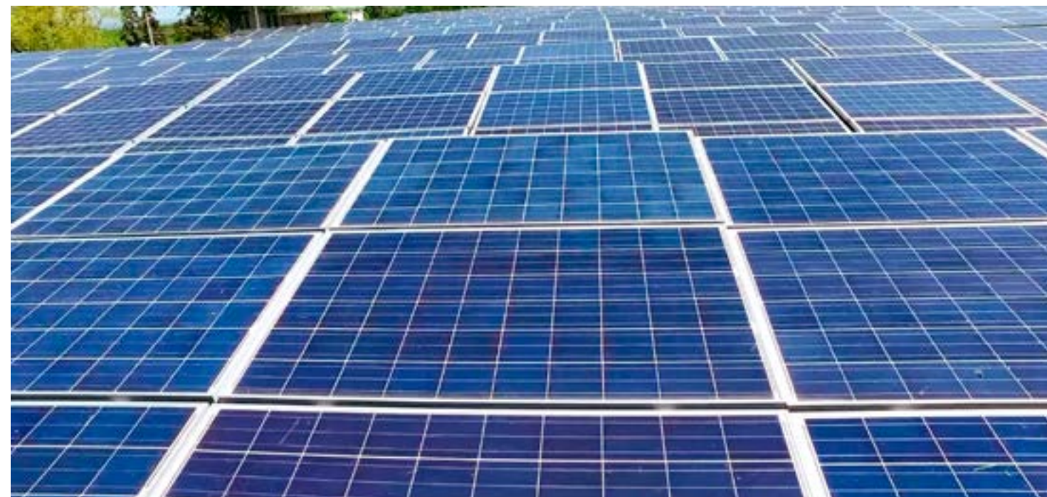
BEVIS HILL SOLAR ARRAY (CITY OF SCHENECTADY)
