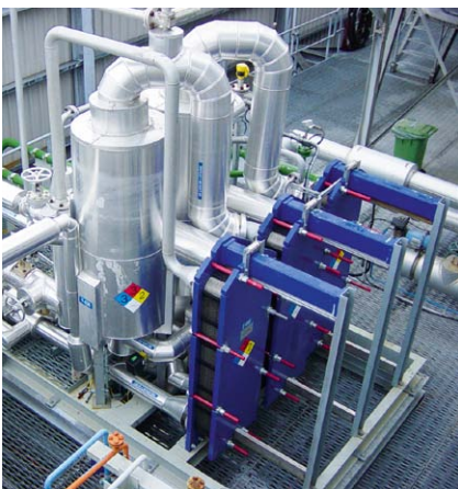
Two-stage evaporation system in a demo plant.
